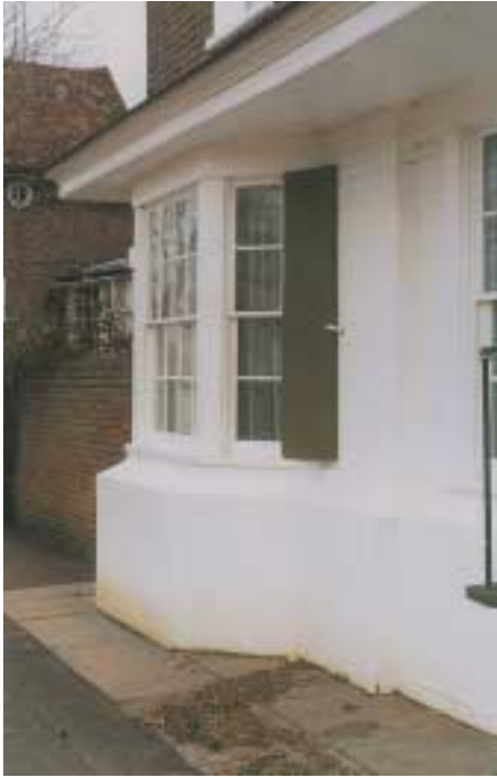
Figure 7 A waterproof render has been applied to the lower external walls of a riverside cottage to form a permanent flood barrier. (John Fidler)
