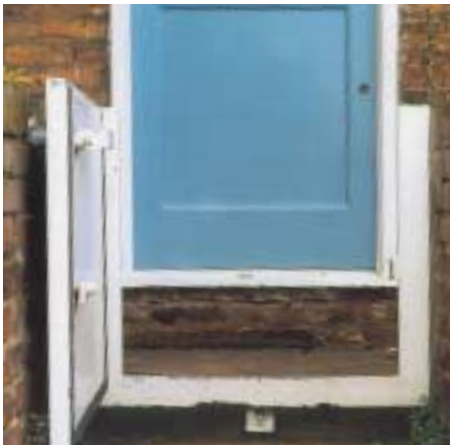
Figure 17 A compression barrier fitted to the front wall of a riverside property that is subject to regular flooding (John Fidler)
